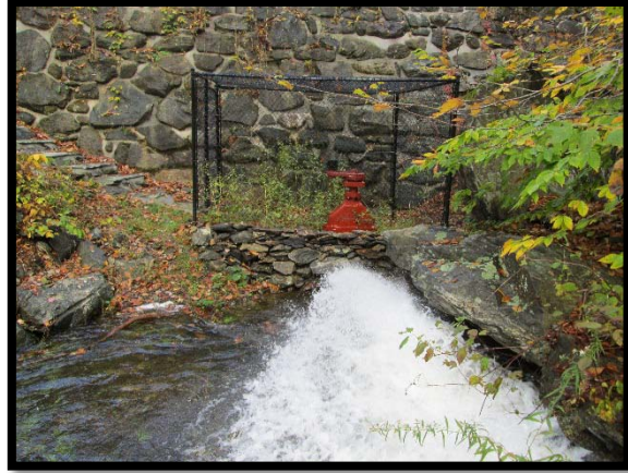
Recently installed low flow drain valve
