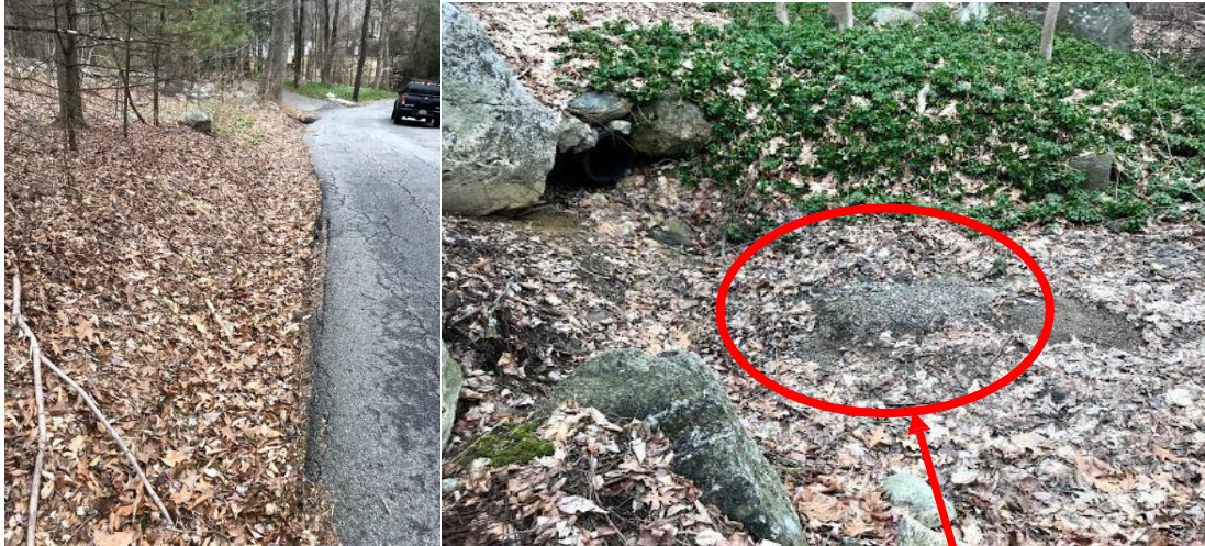
Accumulation of Sediment in Catch
